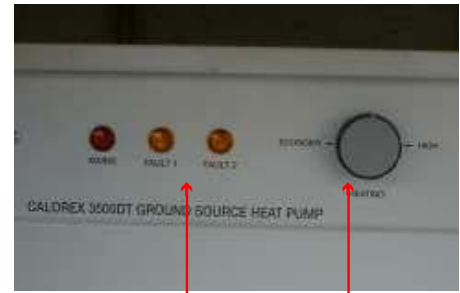
Fault Lights Control Knob
