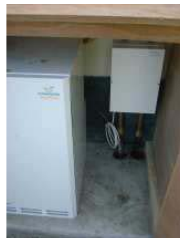
Heat pump as fitted at Chy An Gweal. The heat pump is on the left. The box on the right is the ground loop pump and control box.
