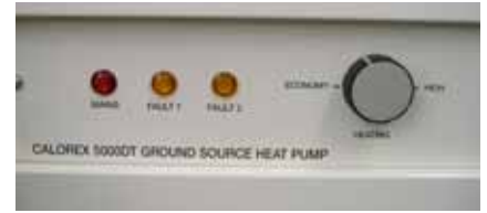
Close up of heat pump front panel showing control knob and fault lights
