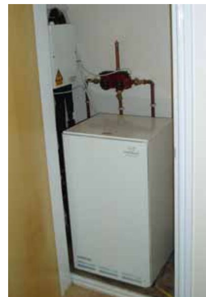
Heat pump with ground loop pump box and heating circulation pump
