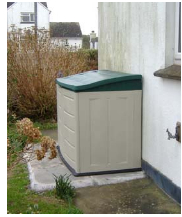
Heat pump outside in weatherproof housing
